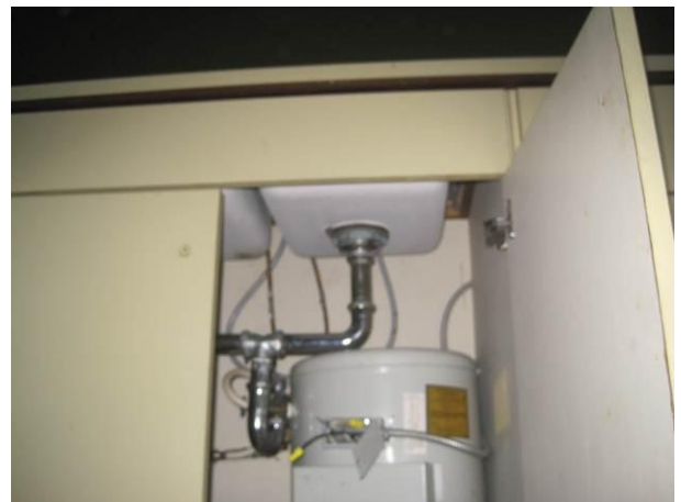
Photo #18 Asbestos-containing Sink Undercoat (White).
