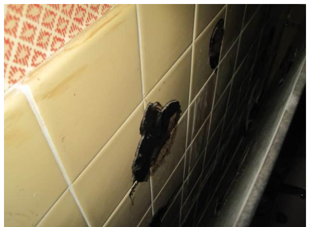
Photo #30 Asbestos-containing Mirror Mastic (Black).
