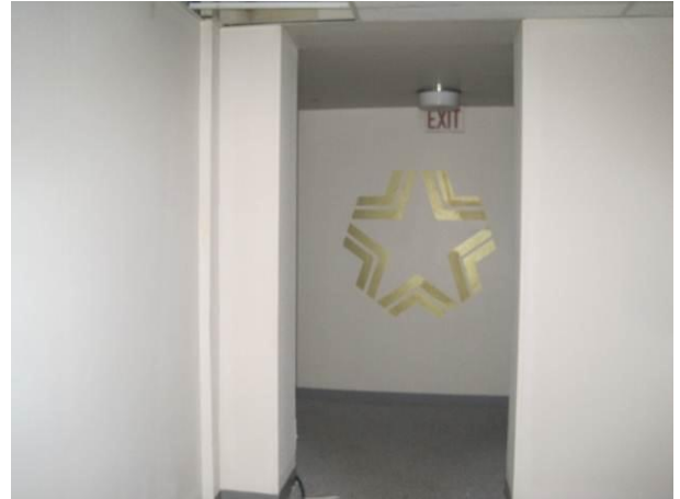
Photo #14 Asbestos-containing Wall Texture / Drywall / Joint Compound (Multicolor, Semi Smooth).
