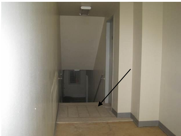
Photo #29 Asbestos-containing 9" x 9" Floor Tile (Tan, 1" Grid Pattern) with Mastic (Yellow).
