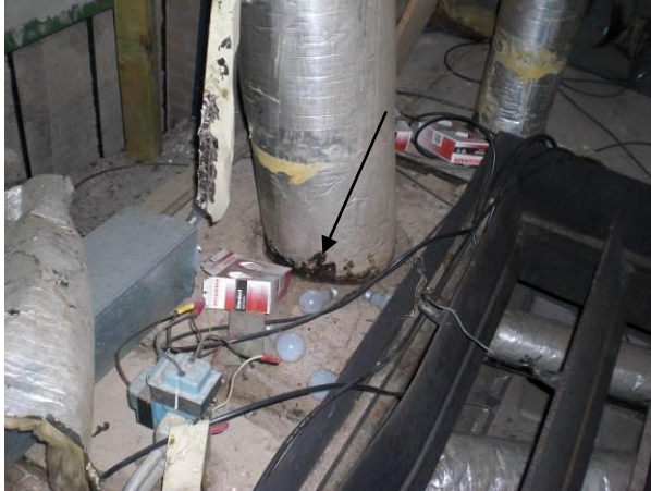
Photo #57 Asbestos-containing Sealant (Black), on Foil Wrap HVAC Duct.
