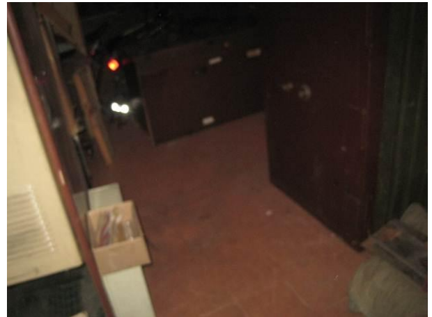
Photo #70 Asbestos-containing Mastic (black) associated with 9" x 9" Floor Tile (Red) with Mastic (Yellow).
