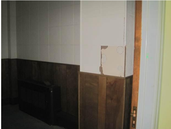
Photo #13 Asbestos-containing Button Mastic (Brown) associated with Acoustical Tile (White, Pinholes).
