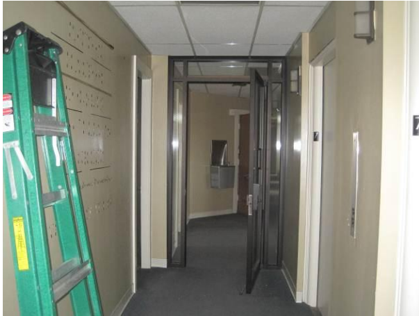
Photo #7 Asbestos-containing Drywall / Joint Compound Associated with Wall Covering (Multicolor).
