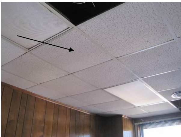
Photo #5 Asbestos-containing 2' x 2' Ceiling Tile (White, Pinholes, Fissures).
