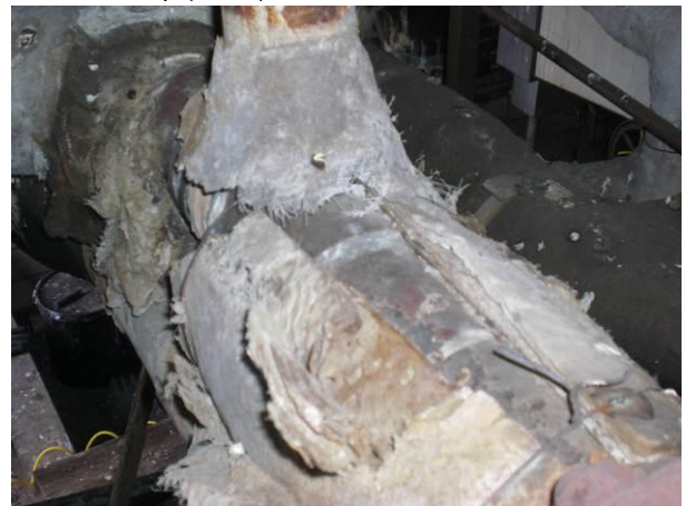
Photo #48 Asbestos-containing Cloth Wrap Aircell Thermal System Insulation Run Insulation (White).
