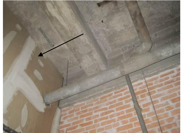
Photo #32 Asbestos-containing Drywall / Joint Compound (Unfinished).
