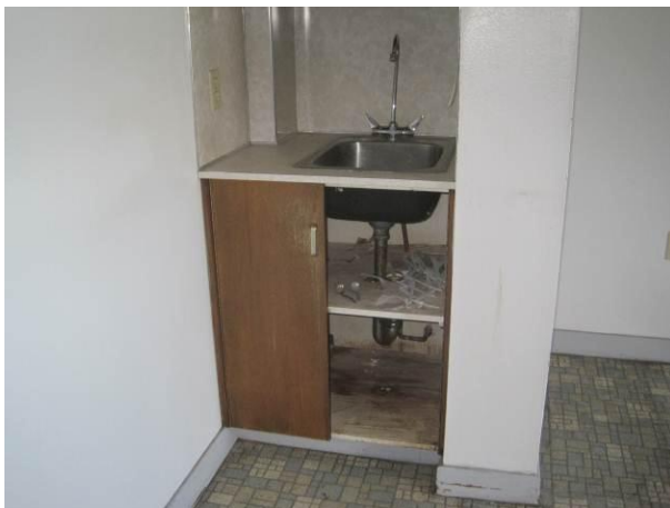
Photo #11 Asbestos-containing Sink Undercoat (Black).
