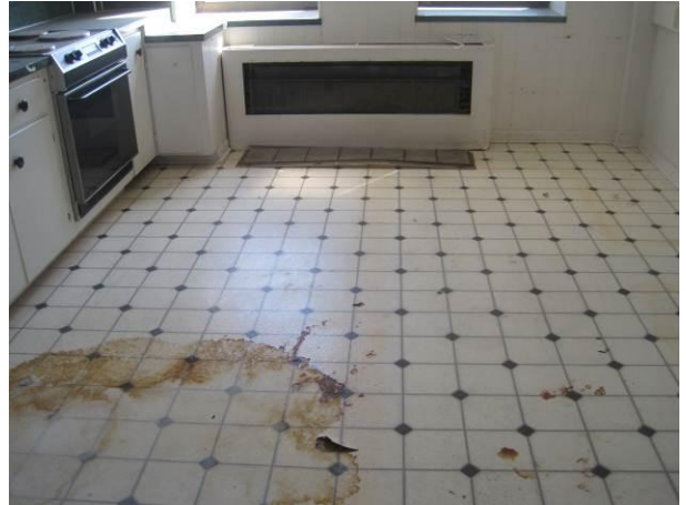
Photo #8 Asbestos-containing Resilient Sheet Flooring (Tan with Black Squares, Multi-Layer).
