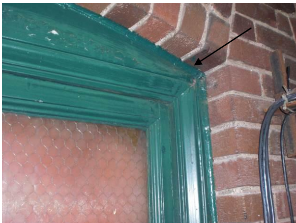
Photo #35 Asbestos-containing Interior Window Caulk (Tan), Associated with Second Floor Air Handler Room.
