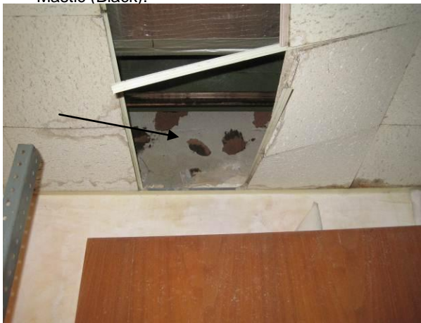
Photo #71 Asbestos-containing Button Mastic (Brown).
