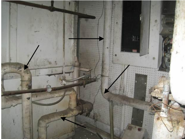
Photo #73 Asbestos-containing Thermal Pipe Insulation (White, Cloth) and Thermal Fitting Insulation (White) Associated with Pipe Insulation (White, Cloth).
