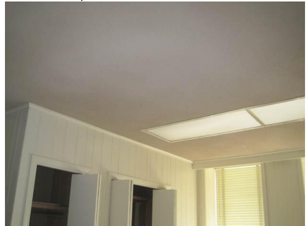
Photo #16 Asbestos-containing Ceiling Plaster (Brown, Rough).
