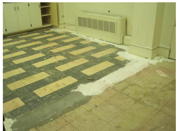
Photo #24 Asbestos-containing Leveling Compound (White) and 9" x 9" Floor Tile (Brown with Tan Specks) with Mastic (Black).
