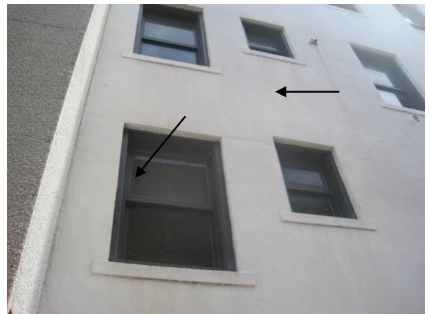
Photo #36 Asbestos-containing Exterior Stucco (Tan) and Exterior Window Glaze (Gray).
