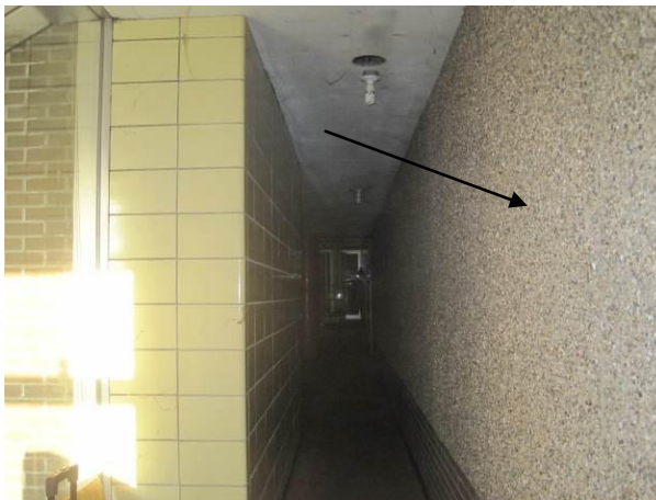
Photo #59 Asbestos-containing Interior Aggregate Cement Panel (Brown).
