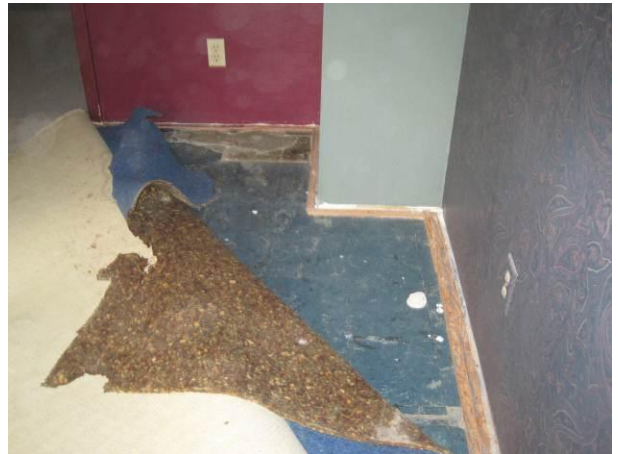
Photo #28 Asbestos-containing 9" x 9" Floor Tile (Blue) with Mastic (Black).
