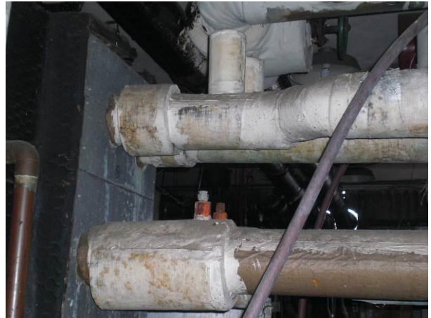
Photo #50 Asbestos-containing Sealant (White, Old) associated with Wrap Fiberglass Thermal System Insulation (White).
