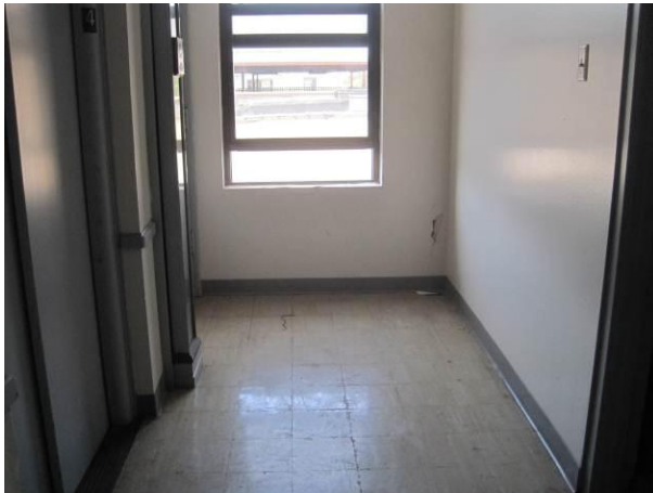
Photo #19 Asbestos-containing 9" x 9" Floor Tile (Tan) with Mastic (Black).
