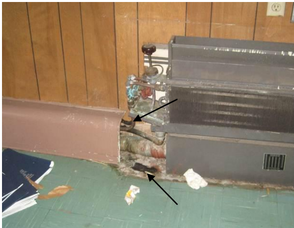
Photo #45 Asbestos-containing Wrap Insulation (Black).
