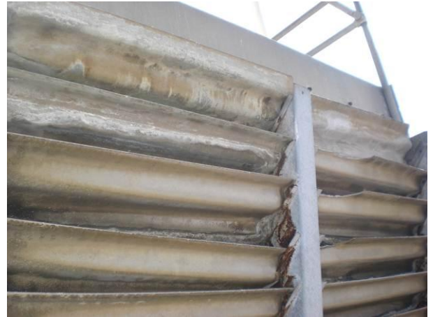
Photo #40 Asbestos-containing 1/8" Corrugated Cementitious Panel (Gray).
