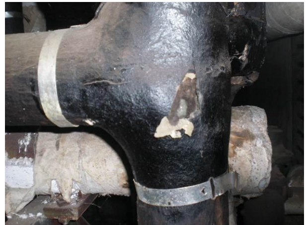
Photo #46 Asbestos-containing Thermal System Insulation Fitting Insulation (Fibrous, Gray) with Tar Wrap (Black).
