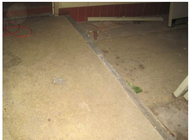
Photo #64 Asbestos-containing Fiber backing associated with Resilient Sheet Flooring (Tan, Rock Pattern) with Mastic (Yellow).
