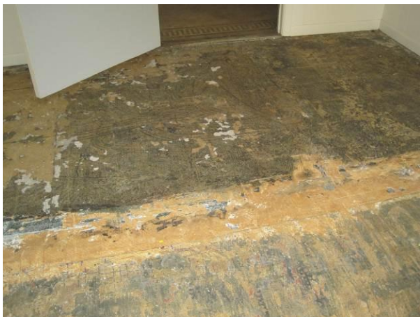
Photo #21 Asbestos-containing Residual Mastic (Black).
