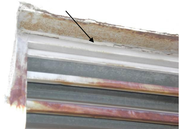
Photo #44 Asbestos-containing Exterior Building Caulk (Gray).
