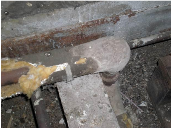
Photo #51 Asbestos-containing Mudded Thermal System Insulation Fittings (White) Associated with Fiberglass Thermal System Insulation Runs.
