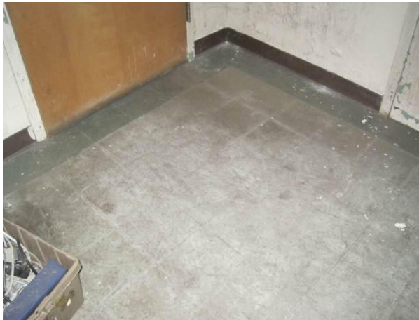
Photo #69 Asbestos-containing 9" x 9" Floor Tile (Tan with Green Specks) with Mastic (Black) and 9" x 9" Floor Tile (Green with Tan Specks) with Mastic (Black).
