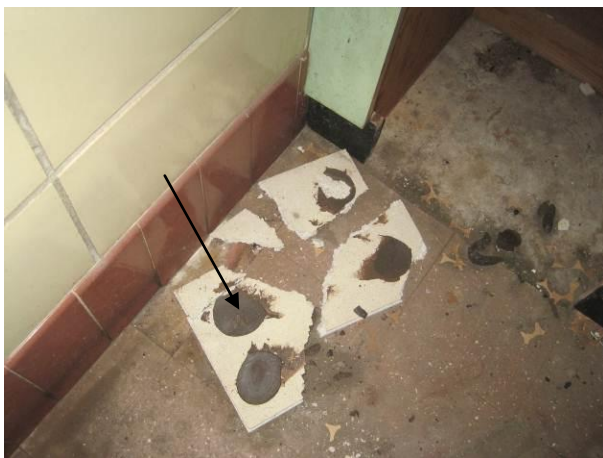
Photo #65 Asbestos-containing Button Mastic (Brown) associated with 1' x 1' Ceiling Tile (White, Pinholes, and Indents).
