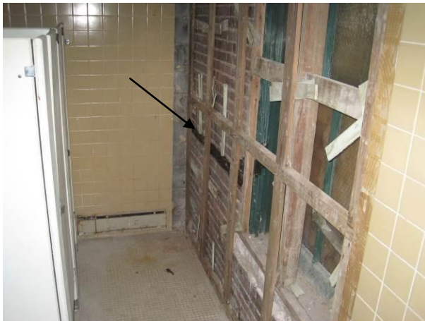
Photo #33 Asbestos-containing Mastic (Black), Associated with Brick Wall.
