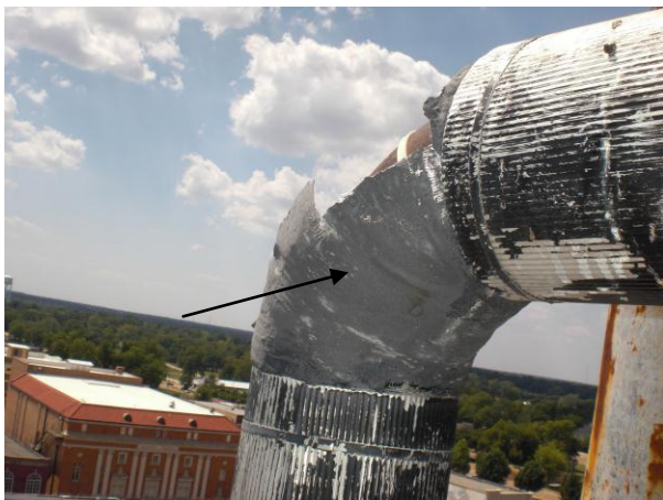
Photo #41 Asbestos-containing Sealant (Gray) on Thermal System Insulation Elbows, Associated with Fiberglass Insulation, under 10" OD
