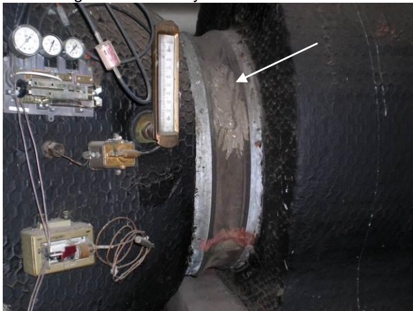
Photo #53 Asbestos-containing Sealant associated with Fiberglass Wrap Insulation (Gray).
