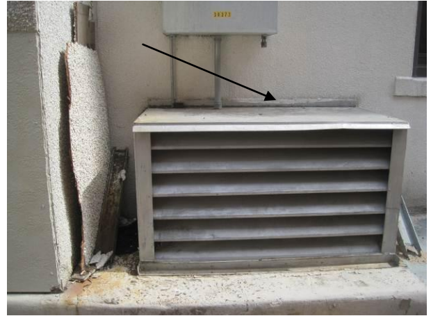
Photo #38 Asbestos-containing Exterior Building Caulk (Black), Associated with Fresh Air Intake.
