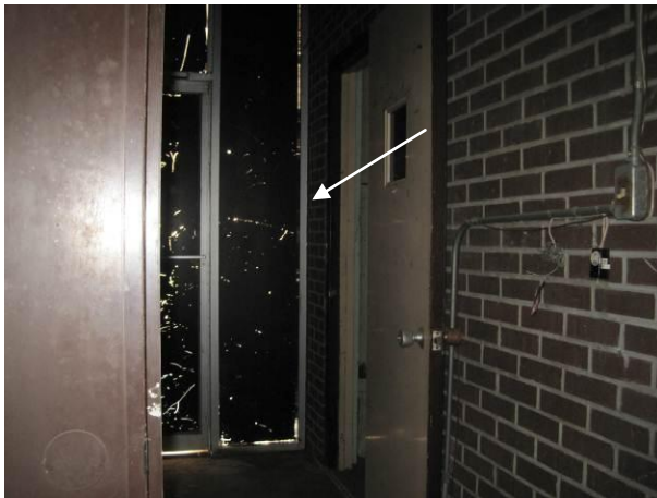
Photo #63 Asbestos-containing Interior Building Caulk (Gray).
