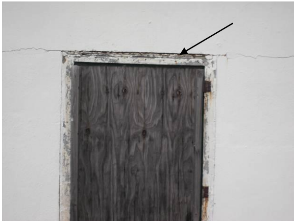
Photo #43 Asbestos-containing Exterior Building Caulk (Gray).
