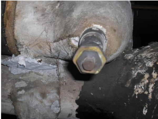
Photo #49 Asbestos-containing Cloth Wrap Mudded Thermal System Insulation Fitting Insulation (White).
