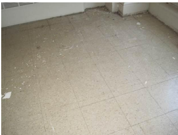
Photo #23 Asbestos-containing 12" x 12" Floor Tile (Brown with Tan / White Specks) with Mastic (Black).
