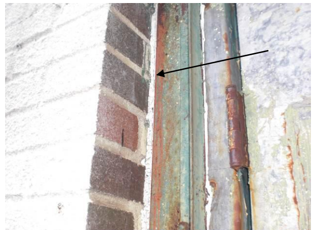
Photo #42 Asbestos-containing Exterior Building Caulk (White).
