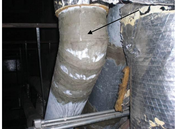
Photo #58 Asbestos-containing Sealant (Green), on HVAC Duct.
