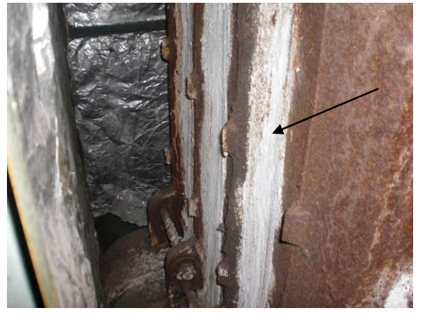
Photo #54 Asbestos-containing Boiler Insulation (White).
