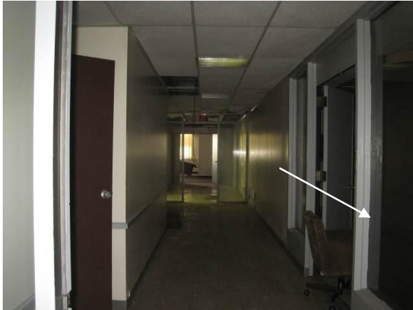
Photo #31 Asbestos-containing Interior Window Caulk (Gray).
