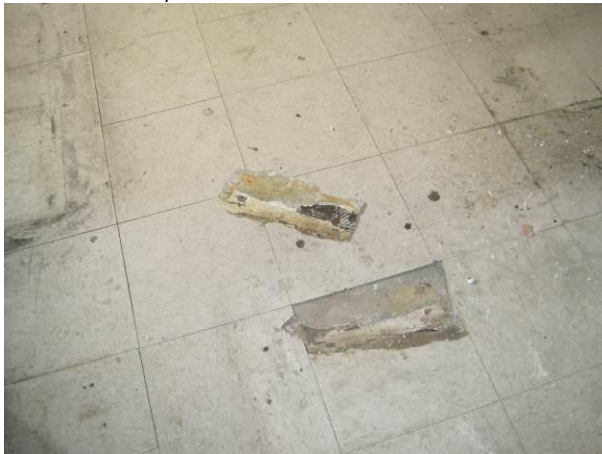
Photo #15 Asbestos-containing 12" x 12" Floor Tile (Tan) with Mastic (Black).
