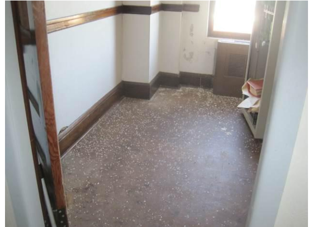
Photo #2 Asbestos-containing 9" x 9" floor tile (brown with tan streaks) and mastic (black).
