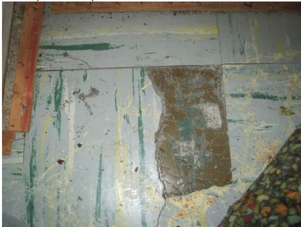
Photo #9 Asbestos-containing Floor Tile Beneath Carpet with Mastic (Black).
