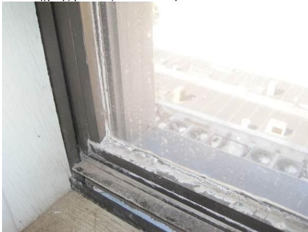
Photo #3 Asbestos-containing interior window glaze (gray).
