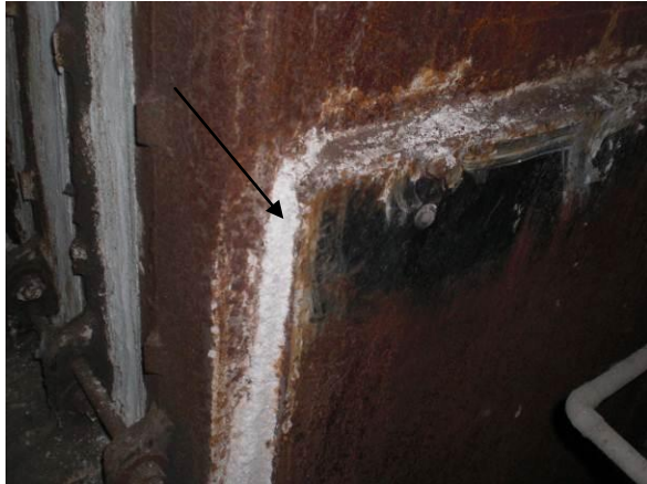
Photo #55 Asbestos-containing Rope Boiler Gasket (White).
