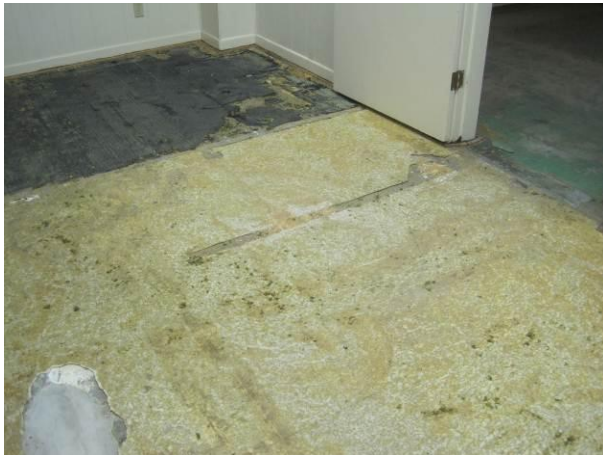
Photo #25 Asbestos-containing Resilient Sheet Flooring (Gray, Rock Pattern).
