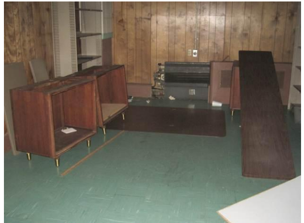
Photo #10 Asbestos-containing 9" x 9" Floor Tile (Green) with Mastic (Black / Brown).
