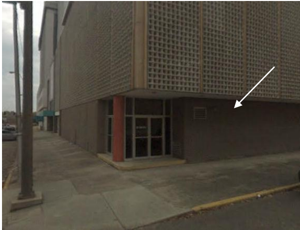
Photo #67 Asbestos-containing Exterior Aggregate Panel (Brown).
