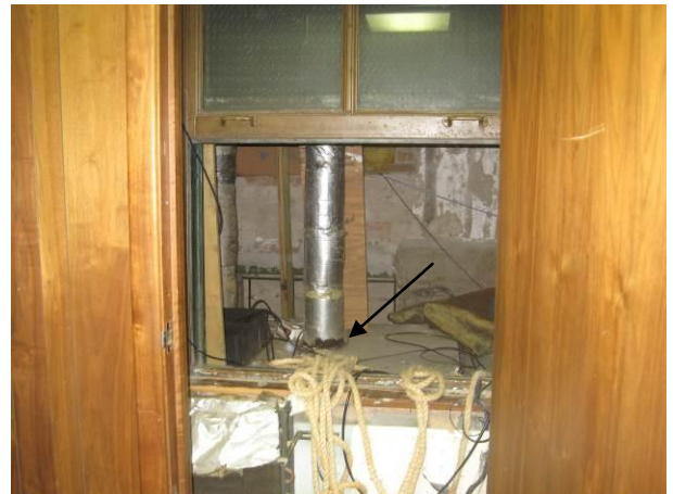
Photo #34 Asbestos-containing Sealant (Black), on Drywall.
