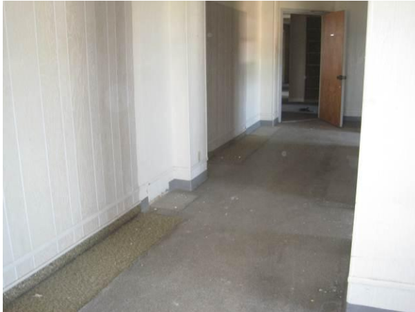
Photo #1 Asbestos-containing floor tile and mastic (black) associated with resilient sheet flooring (gray, pebble, multi-color).
