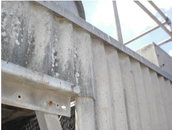
Photo #39 Asbestos-containing 1/2" Corrugated Cementitious Panel (Gray).
