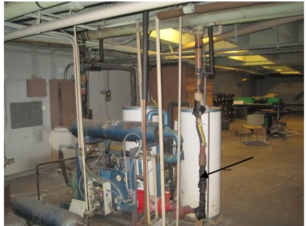
Photo #62 Asbestos-containing Thermal Pipe Wrap (Black).
