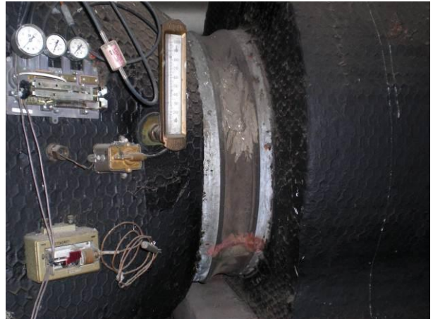
Photo #52 Asbestos-containing Felt associated with Cork AHU Insulation with Tar Coating (Black) with Chicken Wire.
