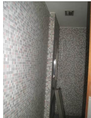
Photo #72 Asbestos-containing Grout (White) Associated with Ceramic Wall Tile.
