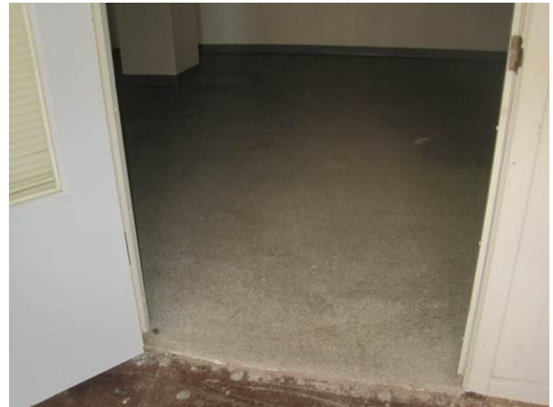
Photo #20 Asbestos-containing Fiber Backing associated with Resilient Sheet Flooring (Gray, Pebble).
