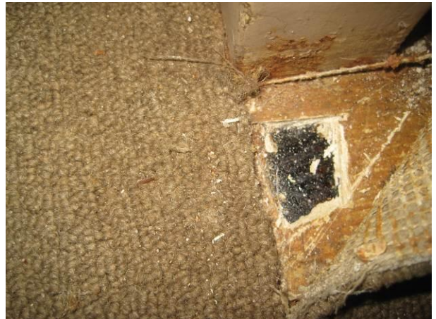
Photo #74 Asbestos-containing Floor Tile (Tan) and Mastic (Black) Beneath Carpet.
