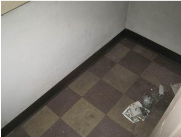
Photo #75 Asbestos-containing 9" x 9" Floor Tile (Brown) with Mastic (Black).
